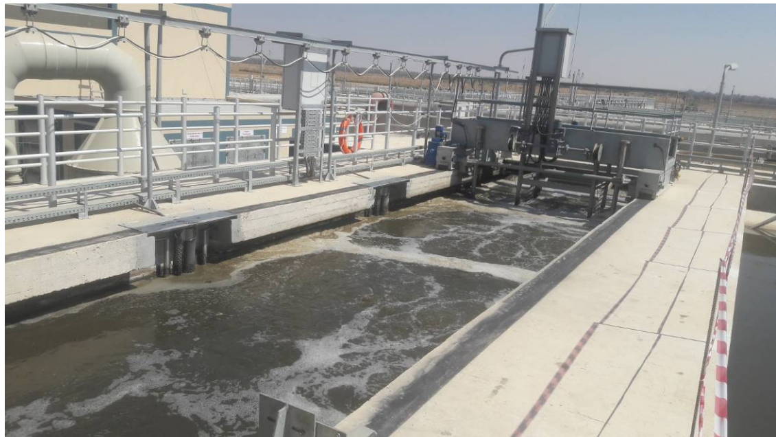
Pre-Treatment Building Filled with Waste Water up to December 2019
