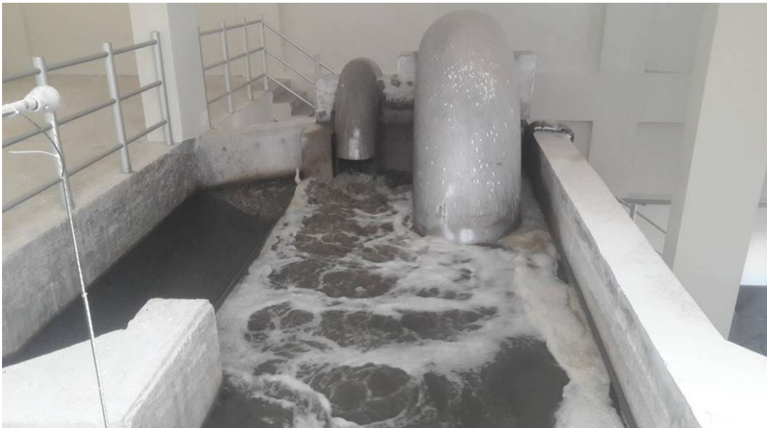
Waste Water Introduced to the Plant from the Inlet Pipe at the Pre-Treatment Building on 09 September 2019
