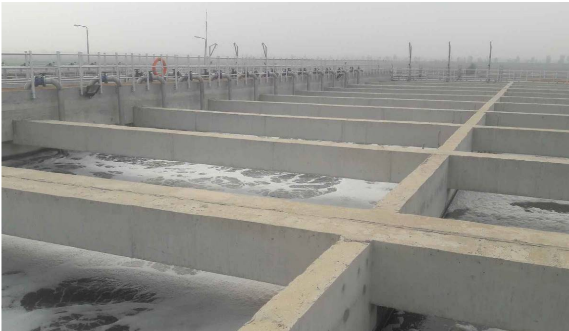
Aeration Tank Filled with Waste Water up to December 2019
