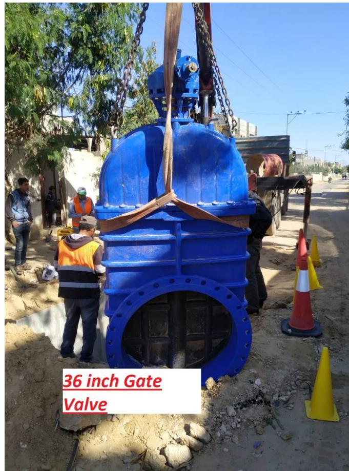
Fittings and Valves entered Gaza and installed on Site for the Effluent Pressure Lines
