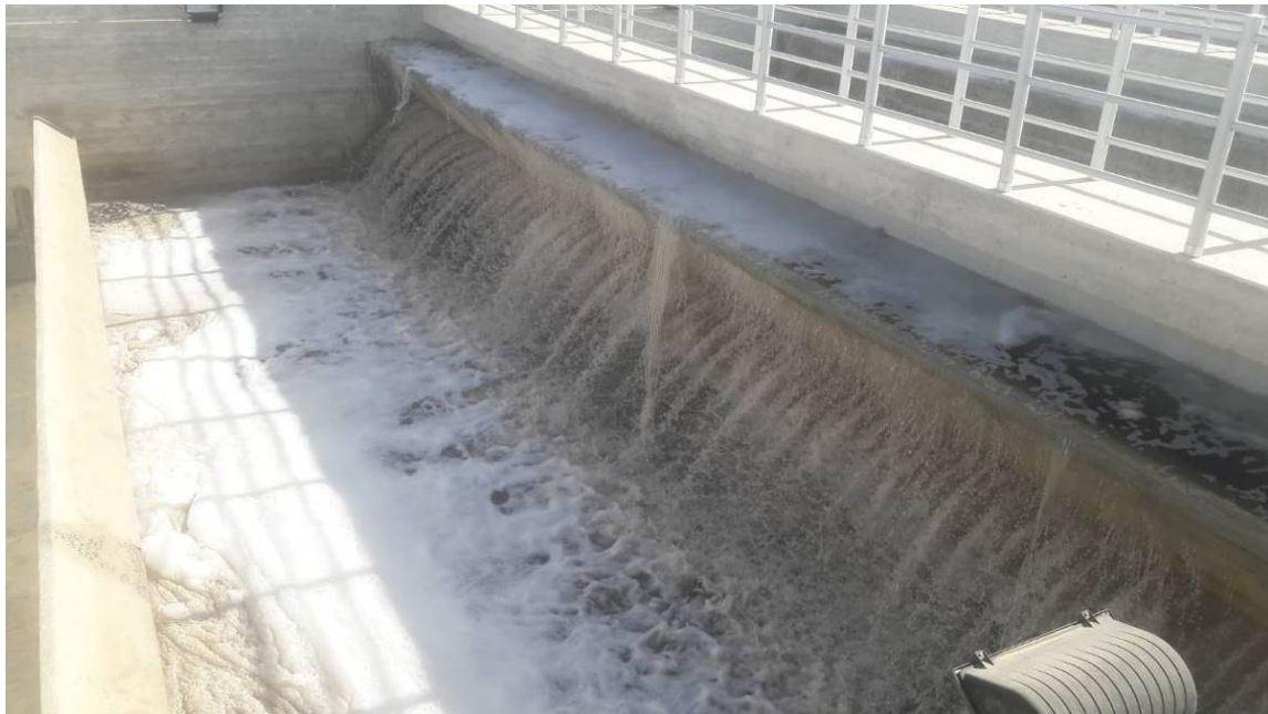
Tertiary Treatment - Purified Water in the Sand Filter up to December 2019
