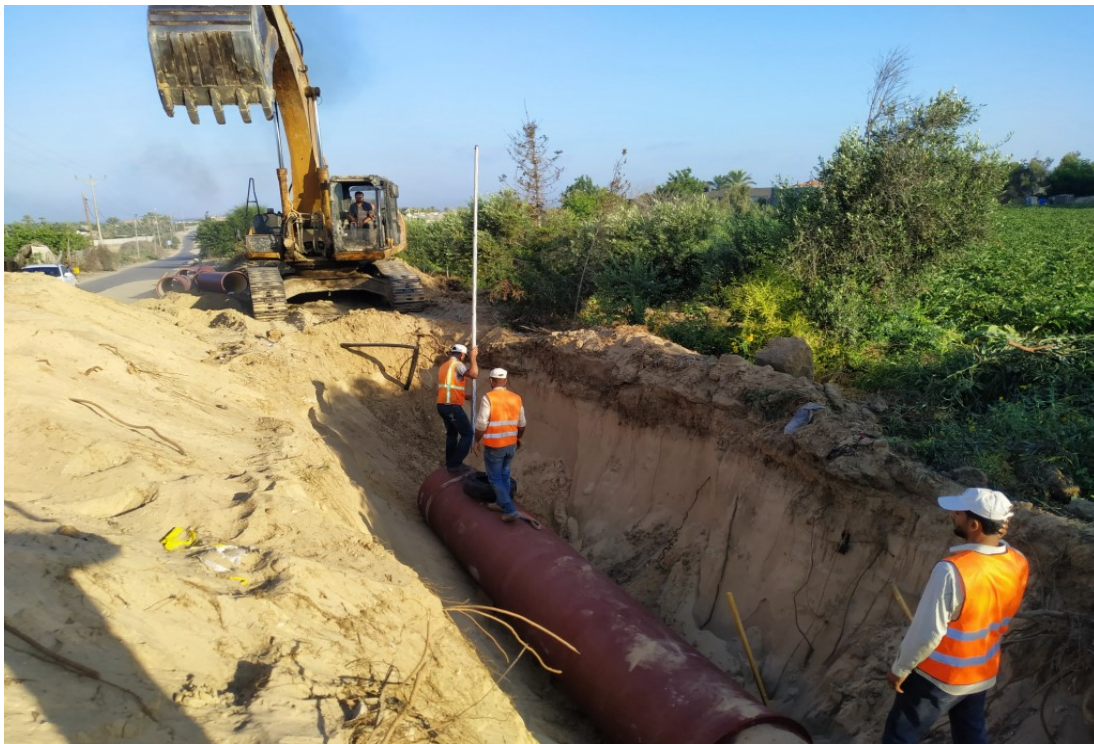
Ductile Iron Pipes Entered Gaza and Installed on Site up to December 2019
